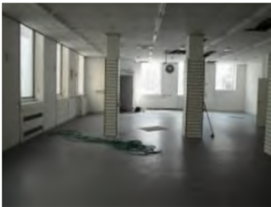
Ground floor illustrating alterations to the plan form and windows (looking east)
