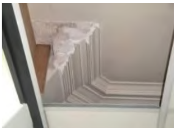
Typical cornice detail and damage incurred by alterations to windows/ installation of suspended ceilings.
