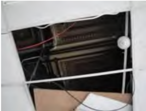
Evidence of damaged moulded plaster ceiling of former Banking Chamber
